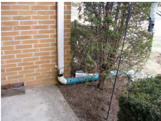
-Disconnected down spout (front of unit)
