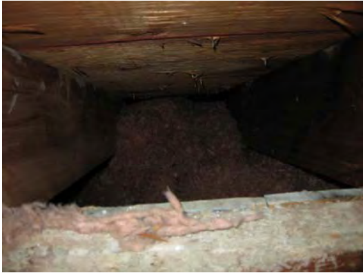
-Blocked joist bay
