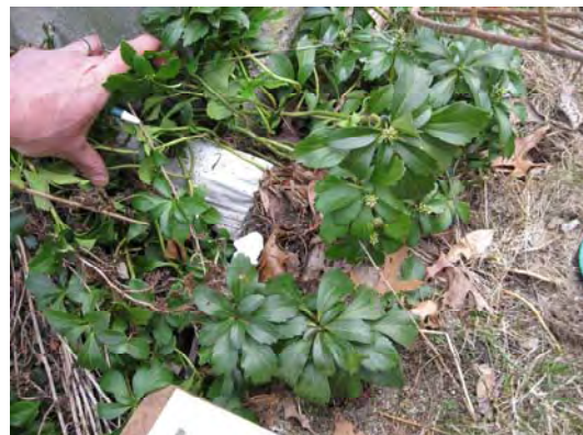
-Blocked downspout (rear of unit)
