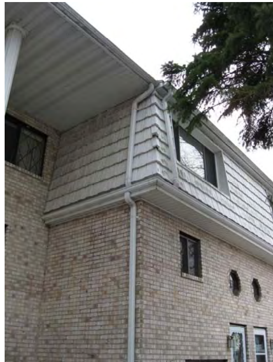
-Hip flashing broken/bent
