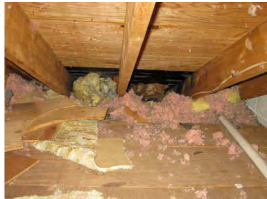
-Blocked rafter bays
