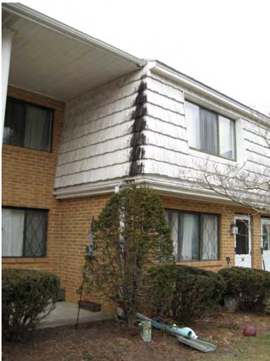
-Missing down spout (front of unit)
