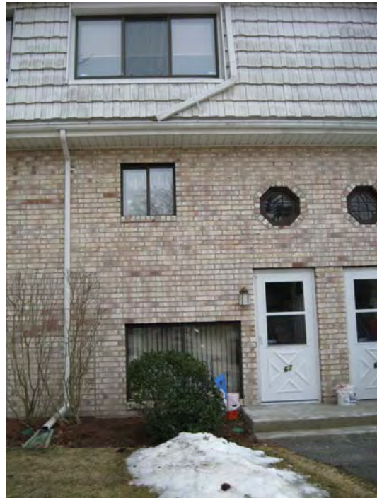
- leaves clogging upper down spout (front of unit)
