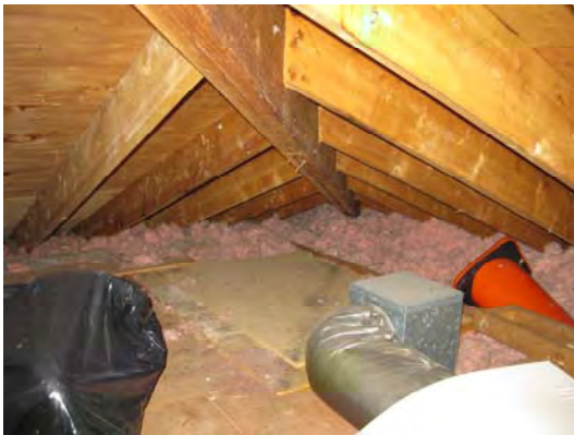
- Blocked rafter bays
