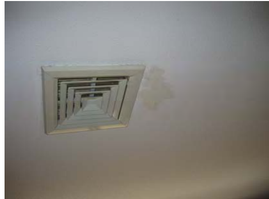
- Water stain on ceiling below turbine vent, wind blown rain possible cause
