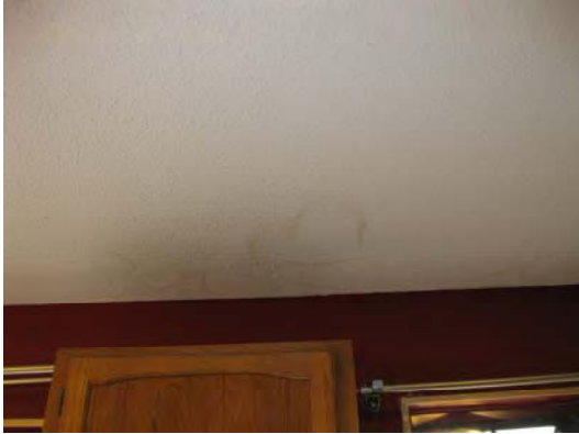
-Stained 1 st floor ceiling (rear of unit)
