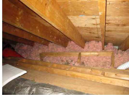
-Blocked rafter bays
