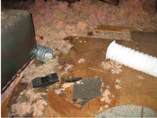
- Bathroom vent disconnected
