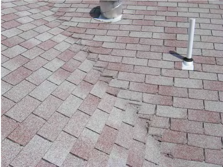
Photograph #10 – Deteriorated Shingles At Woven Valley
