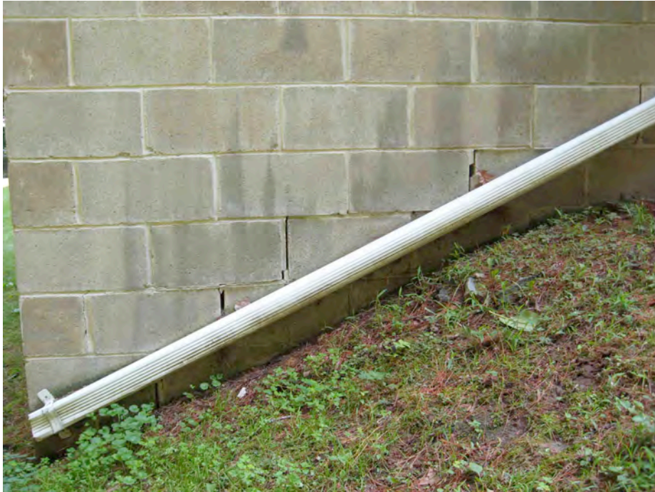
Photograph #6 – Cracked And Displaced CMU Block Wall At Unit 128
