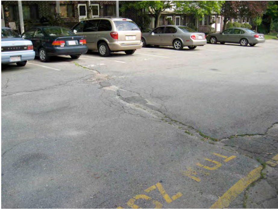
Photograph #1 – Cracked And Settled Bituminous Pavement
