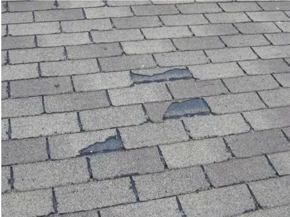
Photograph #12 – Broken Shingle Tabs
