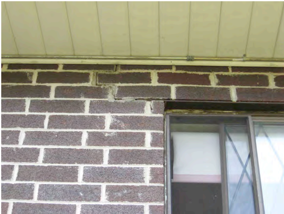
Photograph #2 – Cracked And Displaced Brick Masonry At Lintel End
