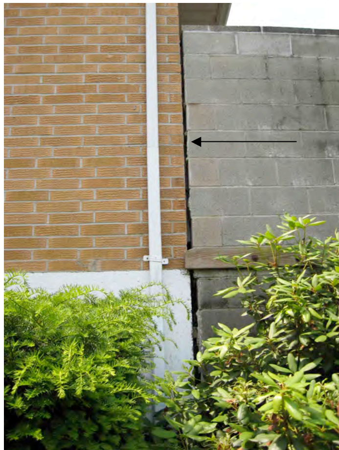
Photograph #7 – Note Gap Between CMU Block Wall And Building Wall
