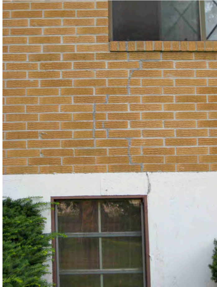
Photograph #3 – Cracking Of Brick Masonry And Foundation Wall
