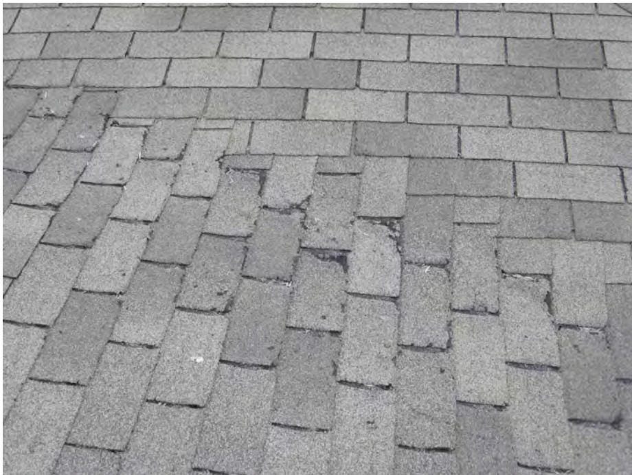
Photograph #11 – Deteriorated Shingles At Woven Valley
