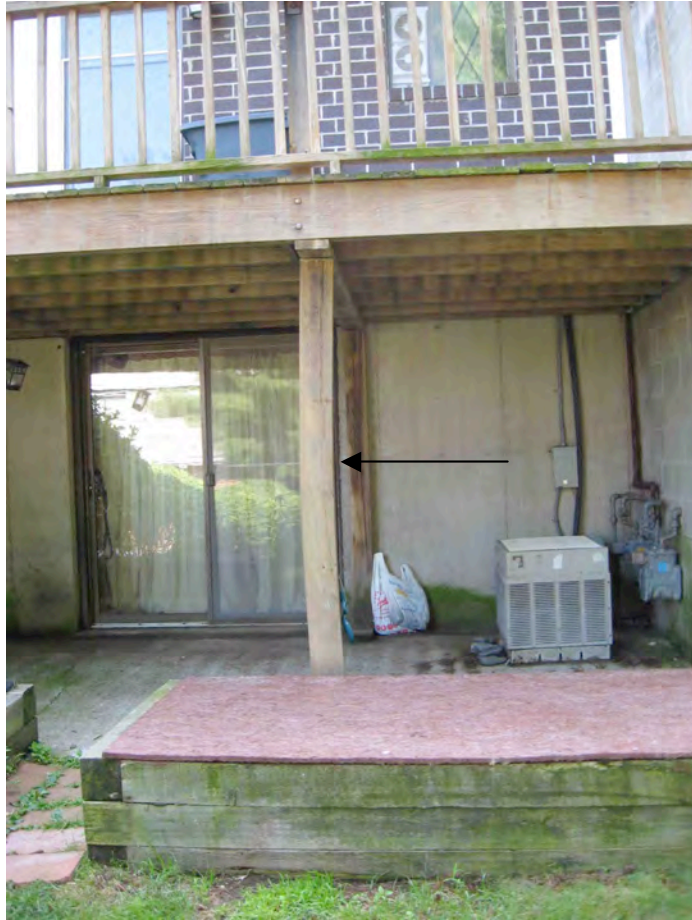
Photograph #4 – Wood Post Below Band Joists At End Unit Deck. Note Bowing Of Post.
